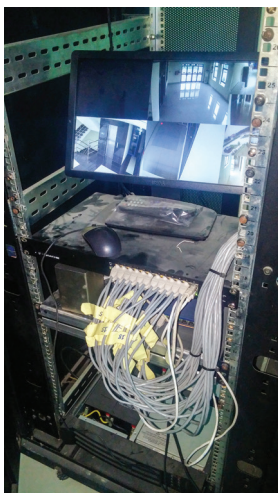
CCTV Cameras recorder
