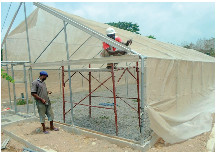
An aeroponics screen house constructed by the Transport section of the institute
